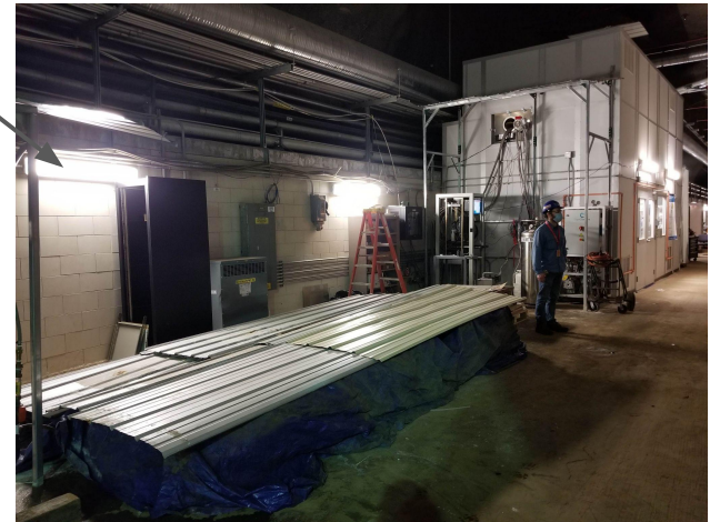
UG site at Fermilab (MINOS)
